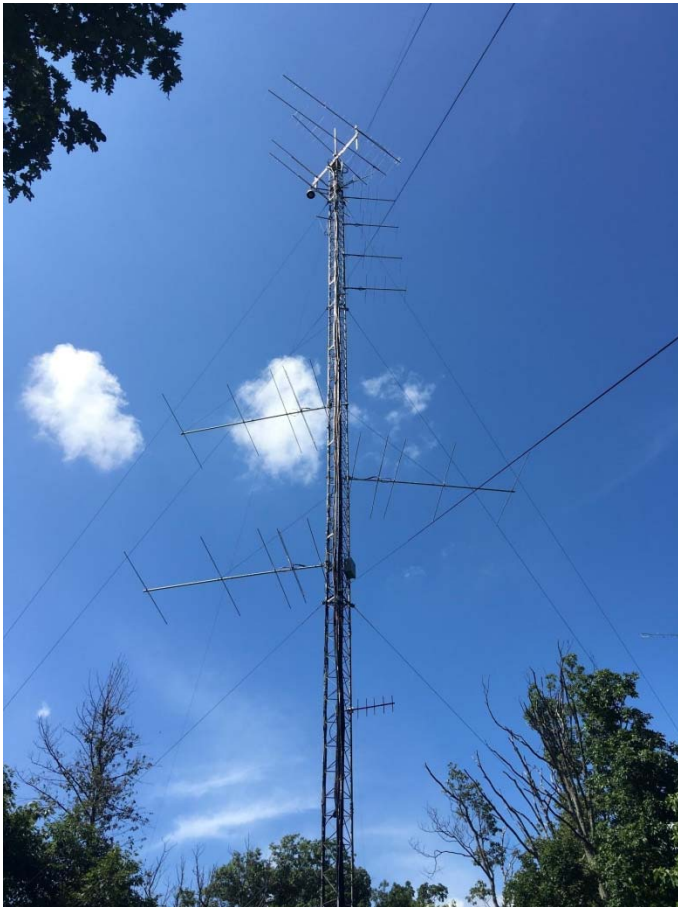
Mike, W3IP's remote setup in FM19 with rotatable array up top and fixed 6 meter and 2 meter arrays. The equipment is in a small enclosure at the base of the tower. (W3IP photo)
